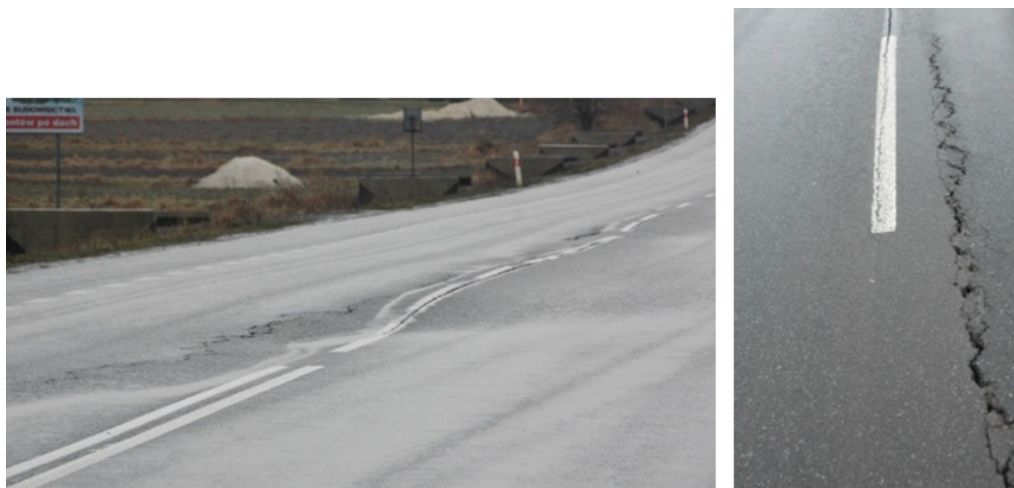
Fig. 11. Corrugations and local depressions of the road pavement (~km 12+750)
