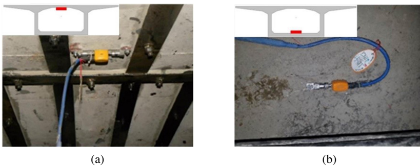
Fig. 14. On-site installation of surface strain gauges: (a) Top slab; (b) Bottom slab
