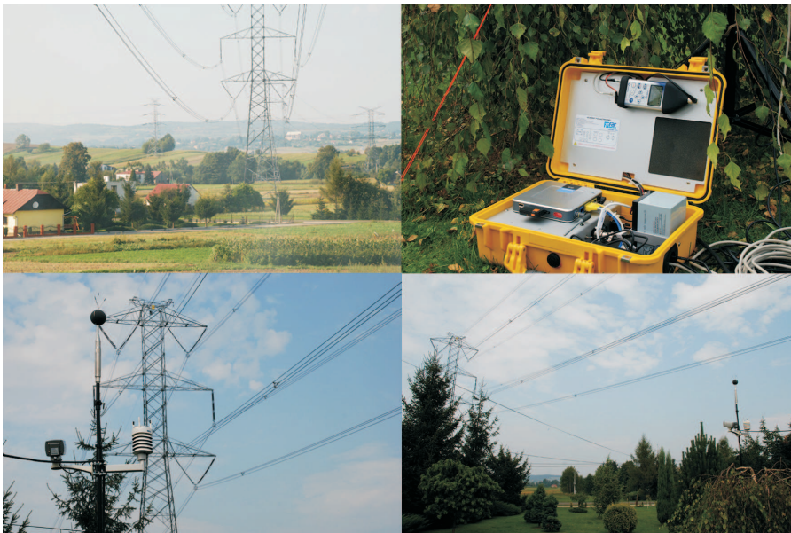
Fig. 3. General view of the acoustic signal continuous monitoring station (ENVIRO131) in vicinity of two circuits of 400 kV power line with triple sub-conductors bundle, 3 \times 350 \text{ mm}^2 .
