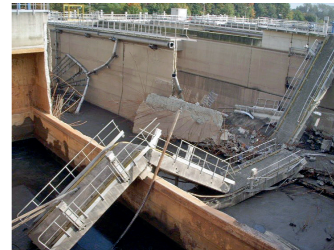
Fig. 8. Collapse of separation wall between full basin at down left, and emptied basin at right
