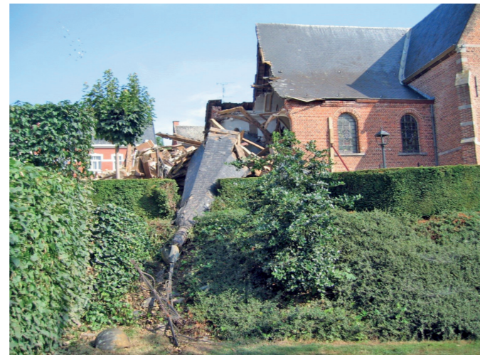
Fig. 11. Collapse of bell tower of St Willibrordus church at Meldert
