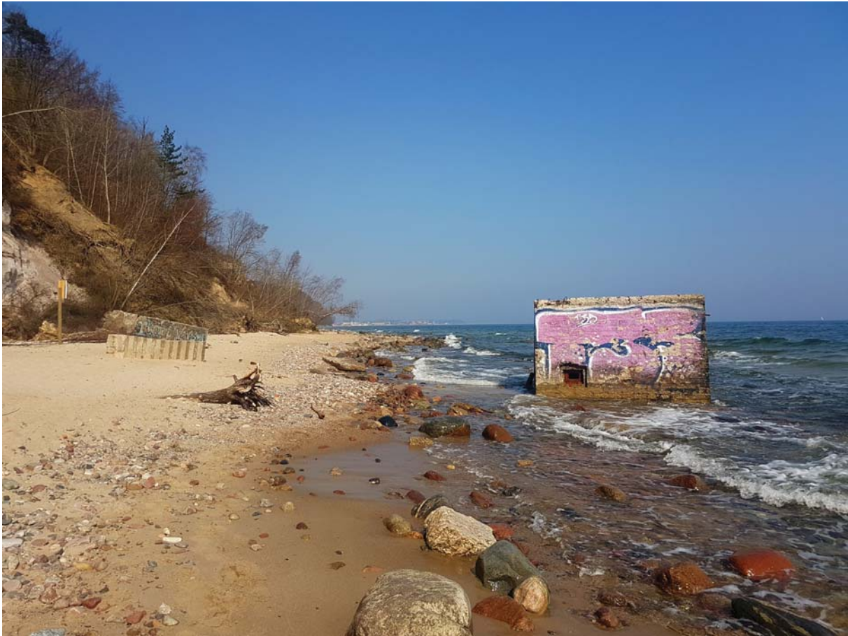
Fig. 8. Two-sided observation bunker after its fall from the Orłowo Cliff (photo by A. Marek).
