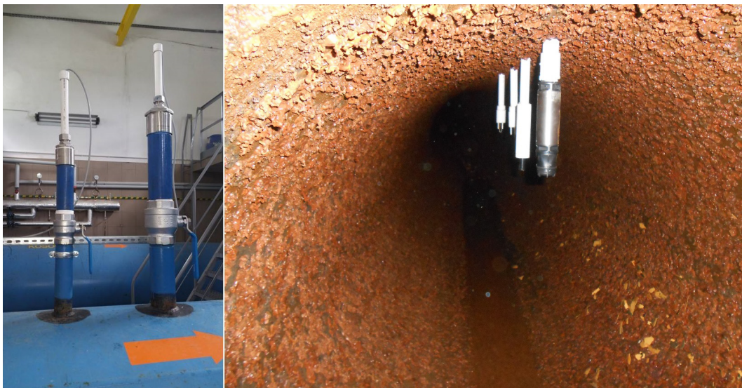
Fig. 2. Assembly of sensors on the left side: view from outside the pipe, on the right side: view from inside the pipe
