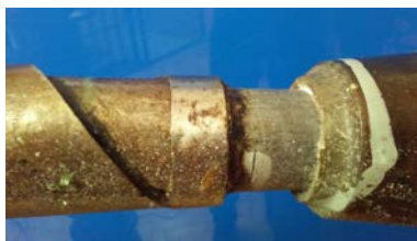
Fig. 2. Investigated cable termination with a partially removed insulating cover of the steel bandage.
