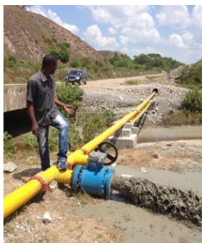
(a) Emergency discharge point
