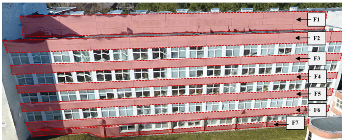
Fig. 10. Linear take-offs of the roof and façade on the basis of the photogrammetry model (source: own study)
