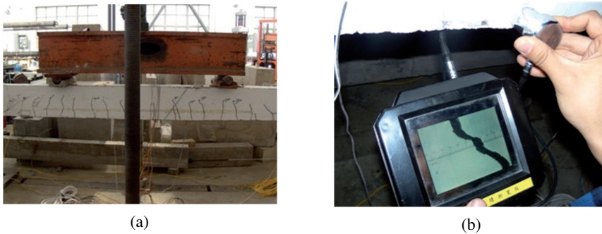
Fig. 15. Distribution and measurement of cracks in prestressed concrete: (a) Crack distribution and (b) Crack measurement
