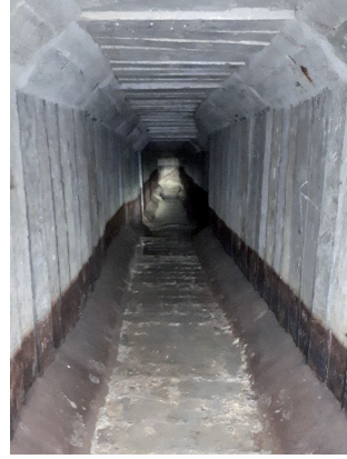
Fig. 10. View of the tunnel running along the northern slope – visible level of maximum flooding of the tunnel (Photo: T. Godlewski, 2022)
