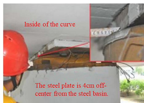
Fig. 7. Slippage of steel plate out of steel pan by 40 mm on bi-directional support
