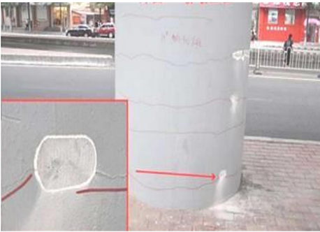
Fig. 8. Semi-circular cracking in the concrete at the base of column
