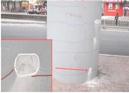
Fig. 9. Bottom half-ring crack in bridge pier concrete
