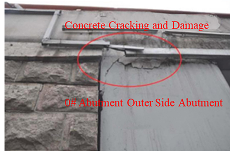
Fig. 36. D0# Abutment outer side abutment top settling and cracking
