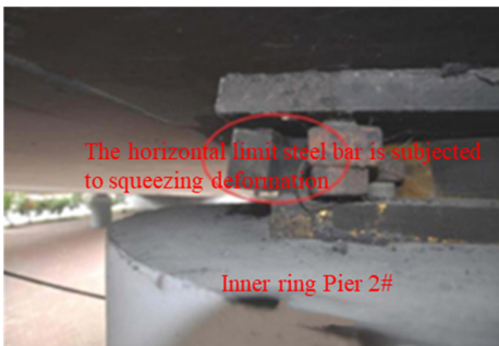
Fig. 6. Compression deformation of lateral restraining steel bar
