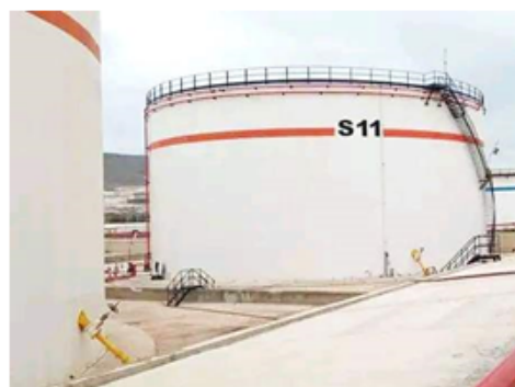
Fig.3. Diesel storage tank S11
