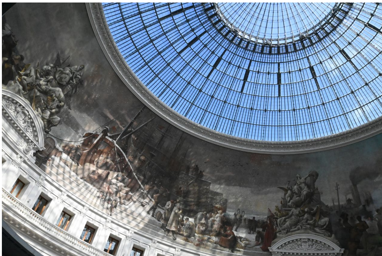
III. 4. Glass dome and reconstructed fresco Triumphal France. Photo by the Author.
