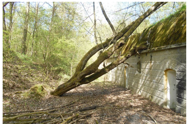
III. 6. Windthrow leaning on a shelter at Fort Parski in Grudziądz, 2018. Photo by the authors.
