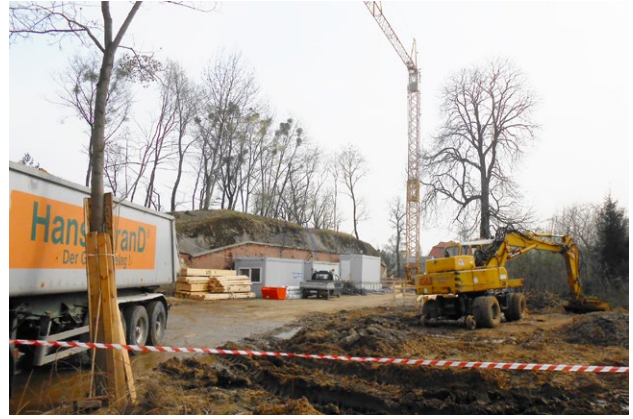
III. 8. Removal of the earth embankment of Infantry Shelter No. 2, Wrocław, 2014. Photo by the authors.
