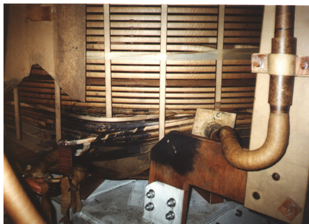
Fig. 4. Deformation of the lower part of the HV winding of the analysed autotransformer
