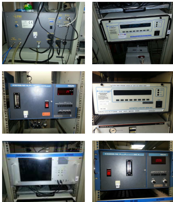
Fig. 2. Equipments used from each monitoring station
