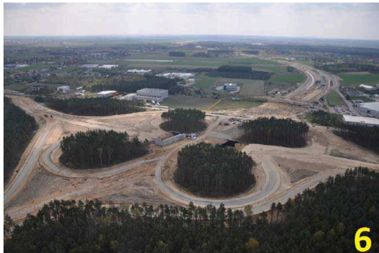
Photo 6. Zakrzewo node under construction – dissection and fragmentation of the forest complex in Zakrzewo region (23.04.2010, A. Kijowski)
