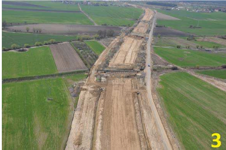
Photo 3. Removal of the humus layer in the ring road of Poznań – dissection of the landscape (23.04.2010, A. Kijowski)
