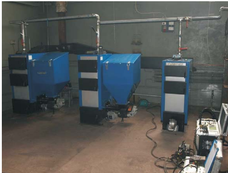
Figure 2. View of testing stand with water boiler of EKO GT – KWR 22 type.
